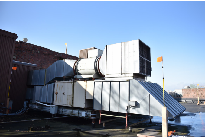
Existing mechanical equipment shown next to flags identifying height at boundary of proposed new Buttnick penthouse
